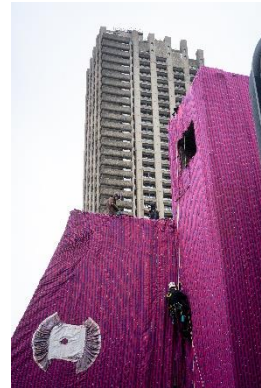
10. Ibrahim Mahama's Purple Hibiscus during installation at the Barbican, 2024. Courtesy Ibrahim Mahama, Red Clay Tamale, Barbican Centre, London and White Cube. © Pete Cadman, Barbican Centre.
