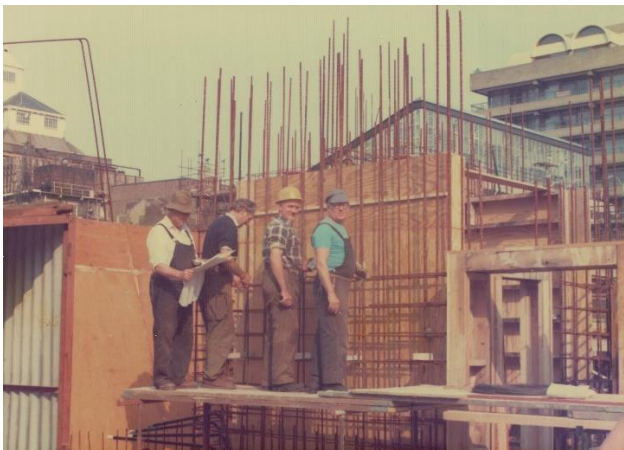
Photograph of Barbican construction workers, captured during the build of the Centre in the late 1970s (Barbican Archive).
